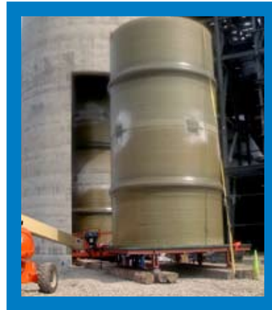
The composite cans were installed into the chimney to form a heat- and corrosion-resistant liner.
